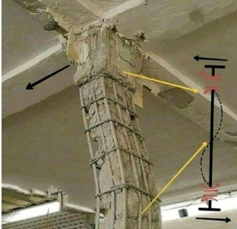
Figure 1.2: Buckling failure in reinforced concrete column
